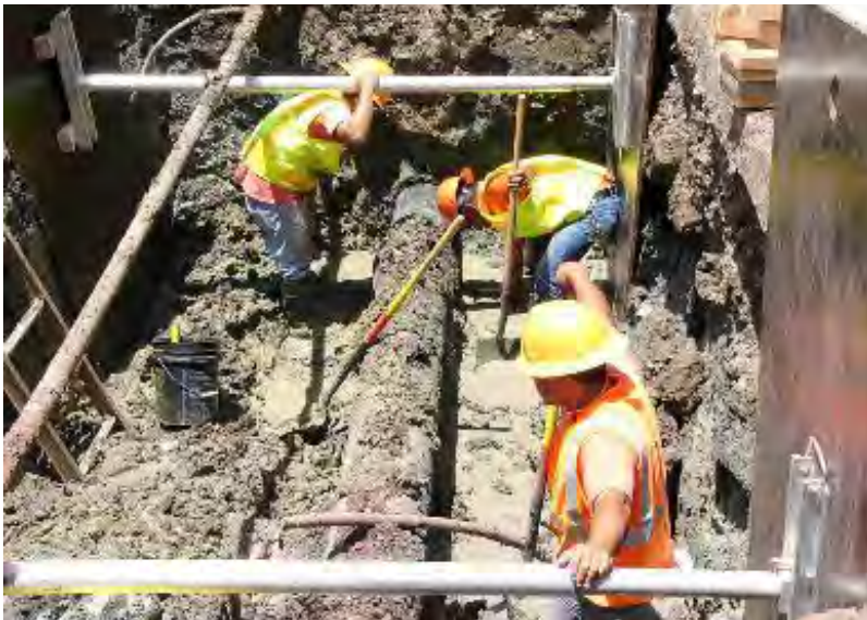
May 2007 Liliha Street main break. BWS crews often work in muddy trenches under bad weather conditions, day and night, to quickly restore water service to customers.
