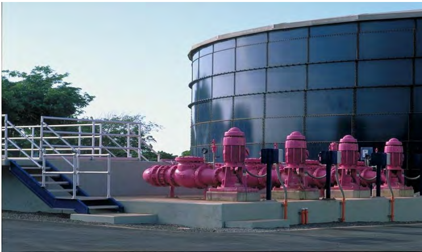
Honouliuli Water Recycling Facility. This BWS facility is designed to generate 12 million gallons of recycled water per day for irrigation and industrial uses.
