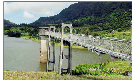
Nuuanu Reservoir No. 4 features a tower which contains three gates or valves which help regulate the water level.
