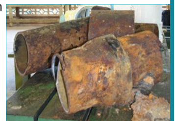
Oahu's soils are highly corrosive and eat away at the pipes.
