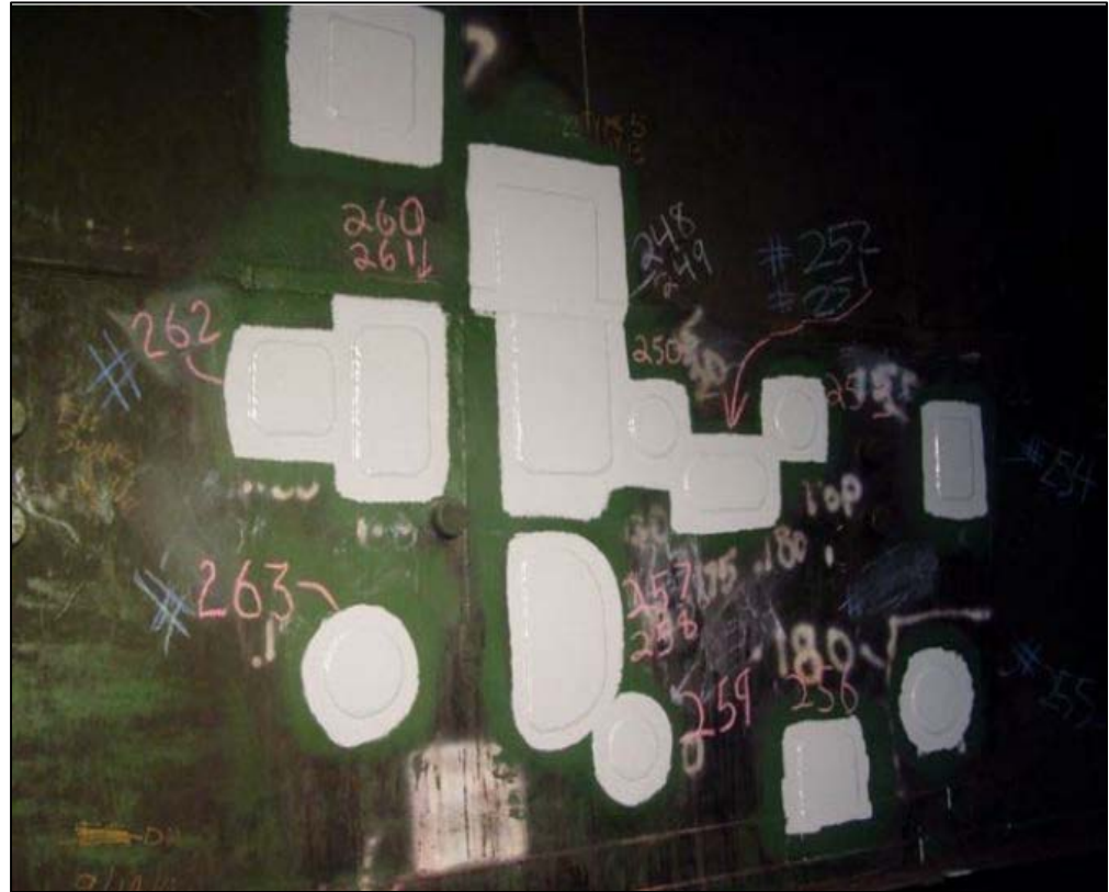
Typical patch plate repairs in Tank 15 Dunkin & Bush Inc., Report on Tank 15 Phase 2 As Built Repairs, Contract number N62742-03-C1402, Clean and Repair Tanks 1, 6, 15, and 16, at Red Hill Fleet and Industrial Supply Center, Pearl Harbor, Hawaii, Dunkin & Bush, Inc., March, 2006 (Navy, 2016).
