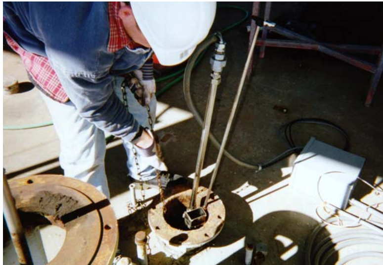
Figure 18. Top of the being installed in an 8-in. opening in a 50,000-gal UST.
