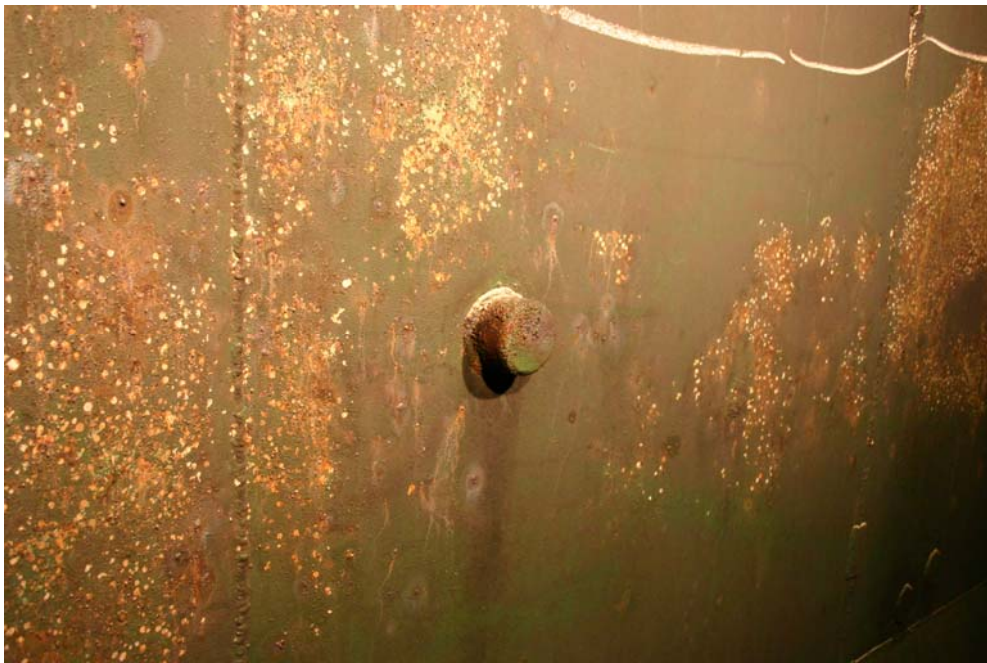
Photograph 6 – A 3-inch grout nozzle that has not been examined by UT testing or eddy current scanning.
