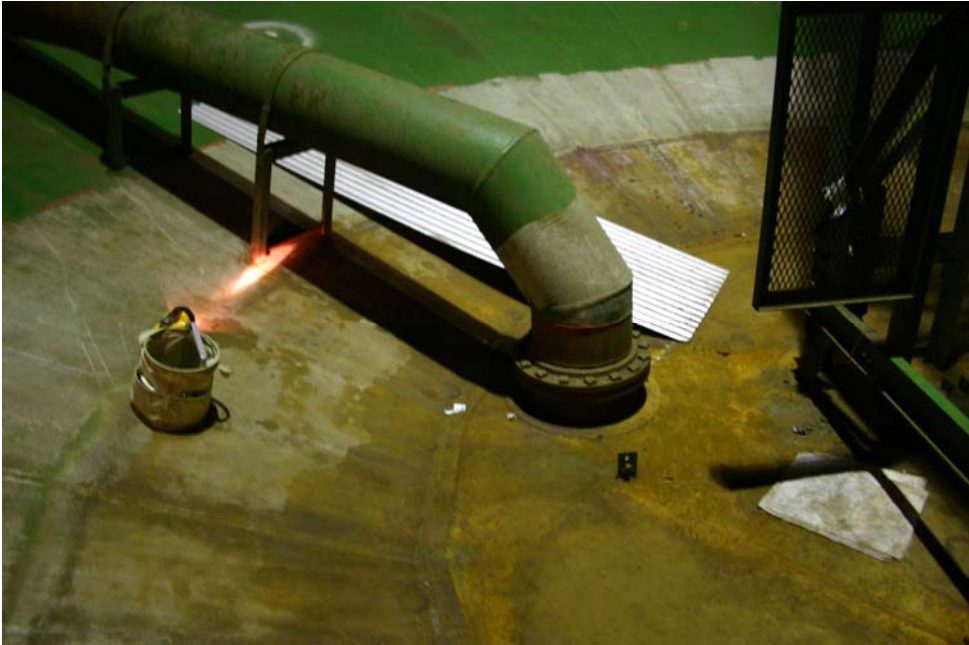
Photograph 8 – The 18-inch inlet/outlet line.
