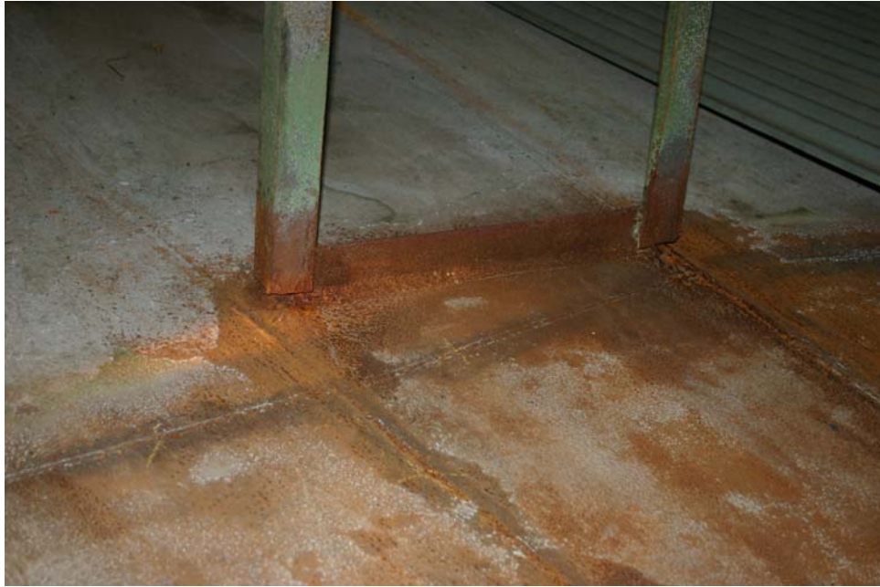
Photograph 7 – Pipe support and reinforcing plate for the 18-inch inlet/outlet line.
