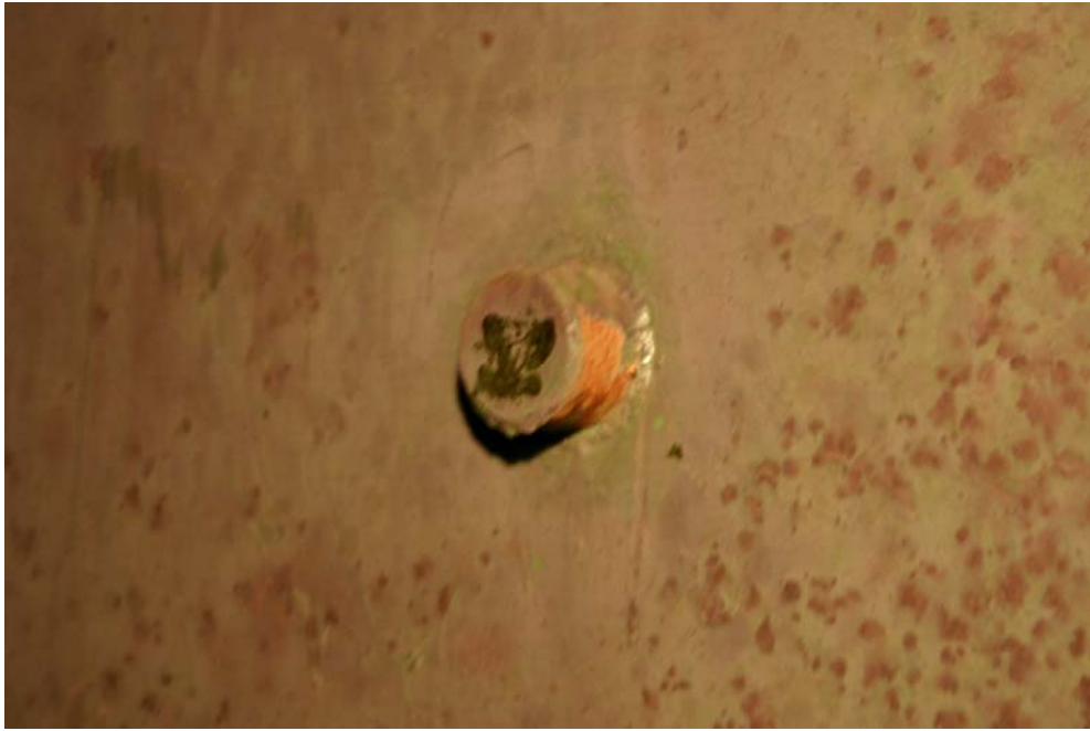
Photograph 5 – A 3-inch grout nozzle that has been examined by UT measurements and eddy current scanning. No weld or metal thickness flaws were detected, however, there is coating failure.
