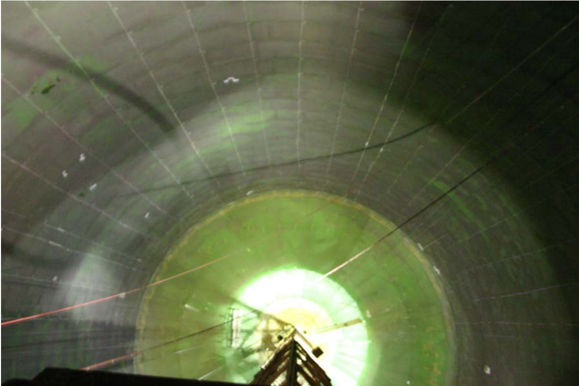
A view from the catwalk looking down at the vertical inspection drops.
