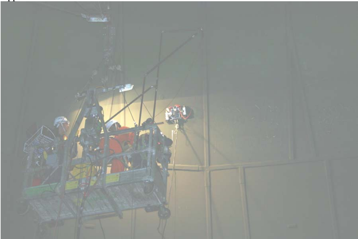
Inspection team #2 using the Viper LFET/U.T. crawler on course C in Quadrant B of the Upper Dome.
