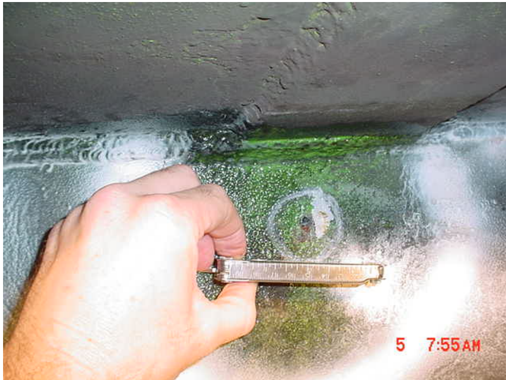
Photograph 1 – Through hole in the expansion joint (Flaw #6).
