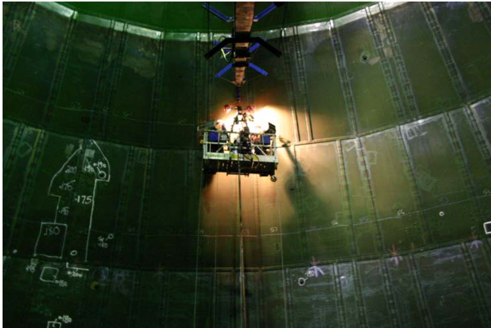
A view of an extensive corrosion area in the upper dome, quadrant C.
