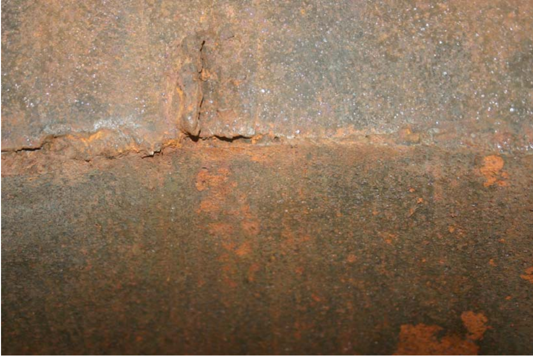
Photograph 9 – Lack of penetration and corrosion on the inside the 32” nozzle at the 45’ station.
