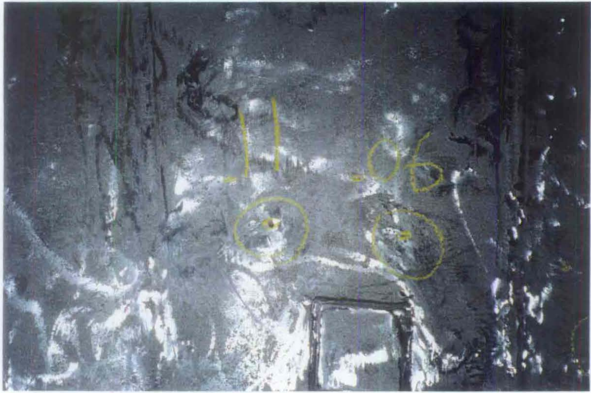
PICTURE OF PITTING ON FIRST ASCENDING PLATES AT BOTTOM OF TANK #10
