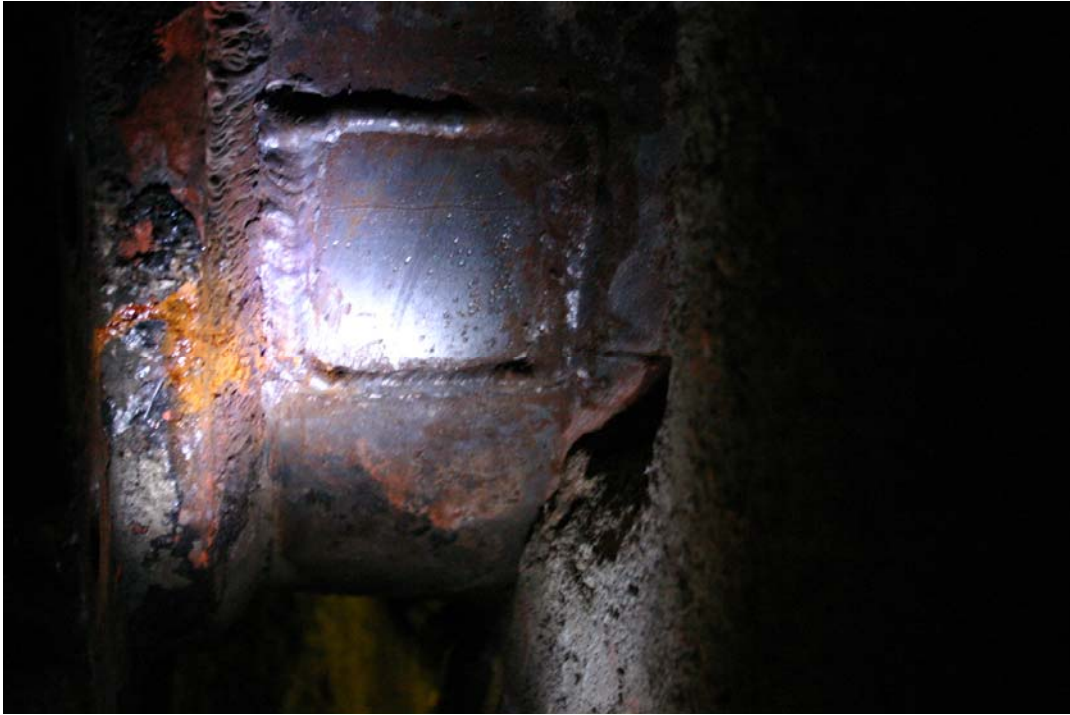
Photograph 11 – A flaw detected by/during the pressure test on the underside of the 32” nozzle that extends into the lower tunnel. The flaw is adjacent to prior repair.
