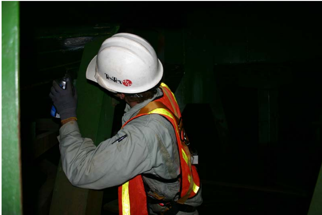
Photograph 6 – NDE technician/examiner painting a flaw indication on course F of the upper dome.
